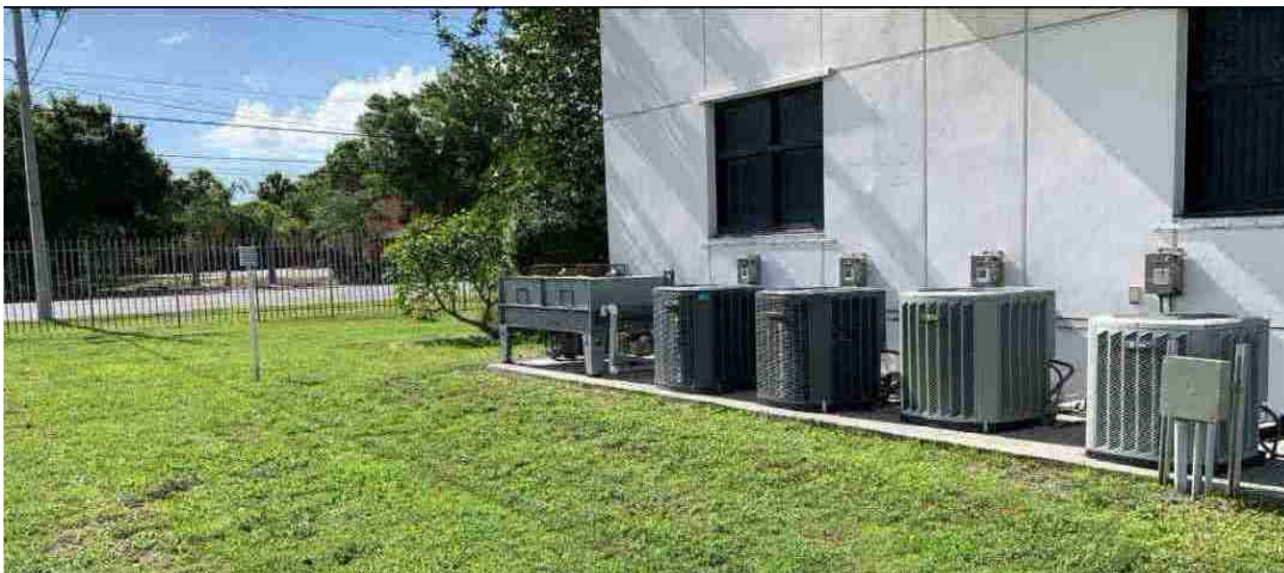
MMTS placement near a building and five air conditioner units at a WWTP, a GHCN station in Fort Pierce, FL. The a/c units produce waste heat, which can easily bias the sensor warmer. Source: Tim Benson.
