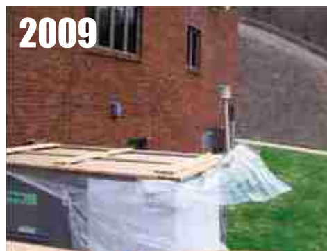
Williamsburg, KY , next to brick building (note the adjacent exhaust vent). RATING = CRN4
