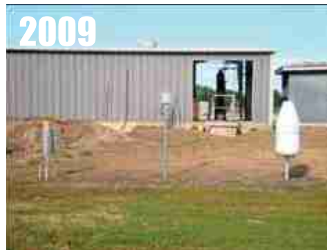
Brinkley, AR , nearby building with 3 air blowers, dirt mound, raw sewage at WWTP. RATING = CRN3
