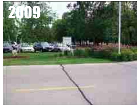
Milwaukee, WI , nearby road. RATING = CRN4
