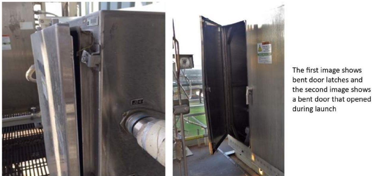
Figure 6: ML-1 Panel Door Damage Post-Artemis I Launch
